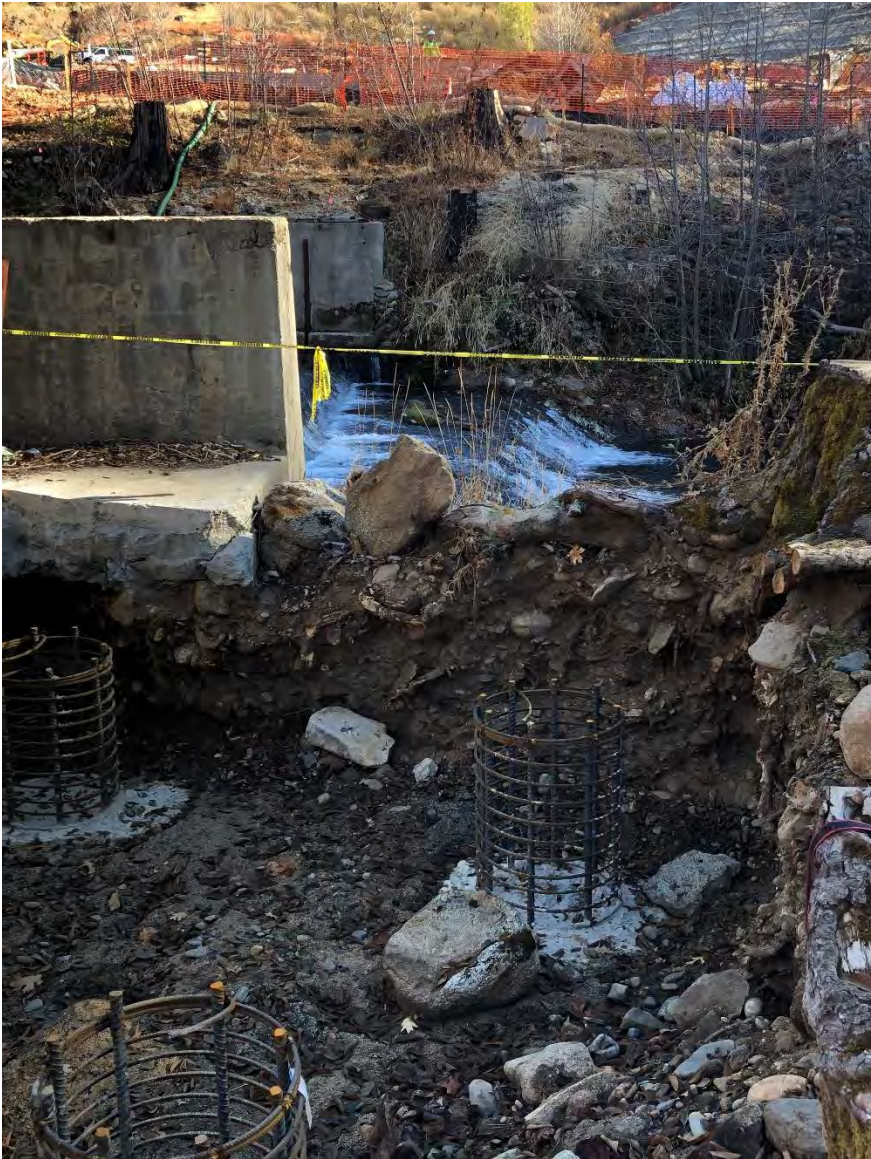
Construction progress for pier of pedestrian bridge over the South Fork Tuolumne River
