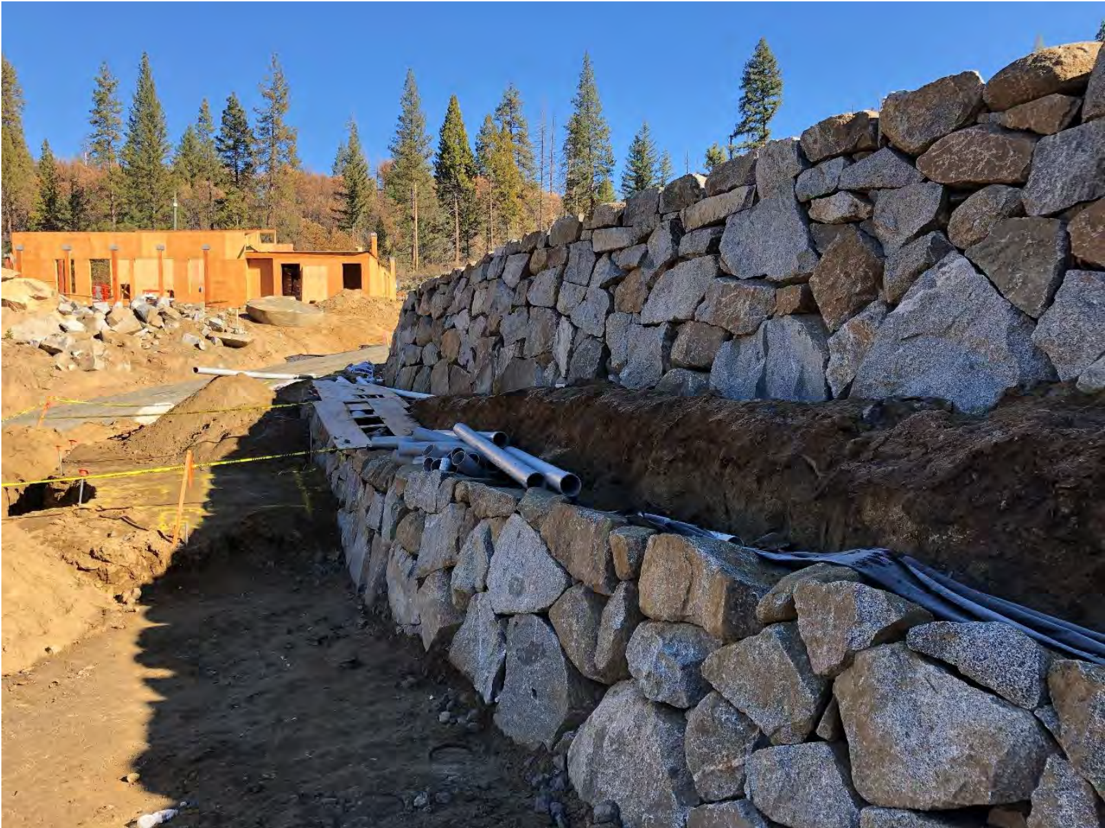
Rock Retaining Walls (all rock is from on-site, Recreation Hall in left background)
