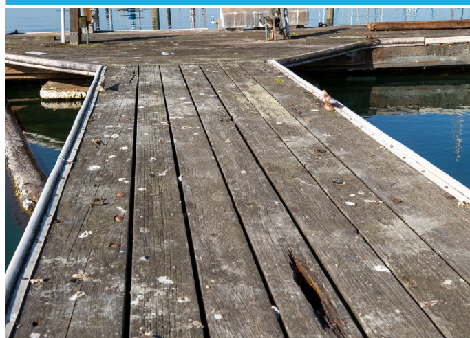
Deteriorated Marina Dock
