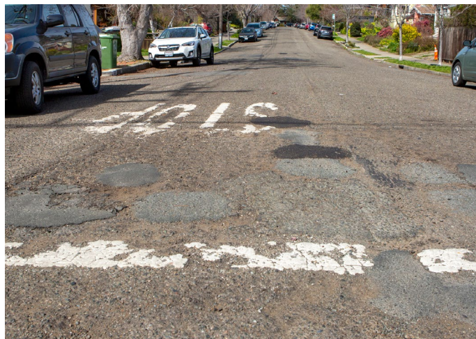
Street Pavement Damage
