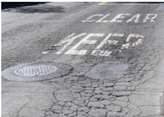
Street surface in need of repairs
