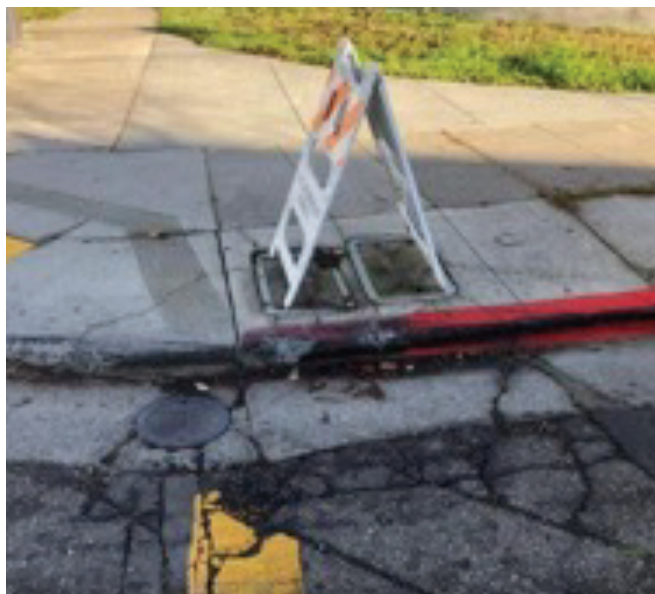
Sidewalk tripping hazard
