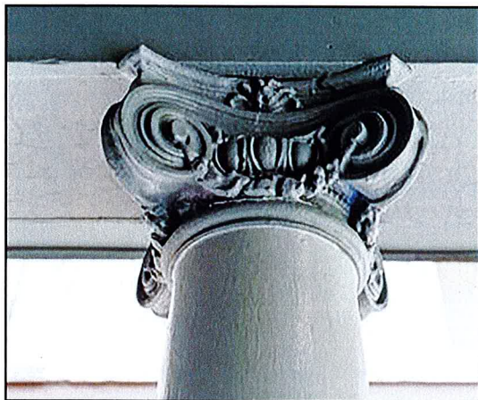
Fig. 8. An Ionic capital on a porch column. The Grubb Company listing photo, 2021
