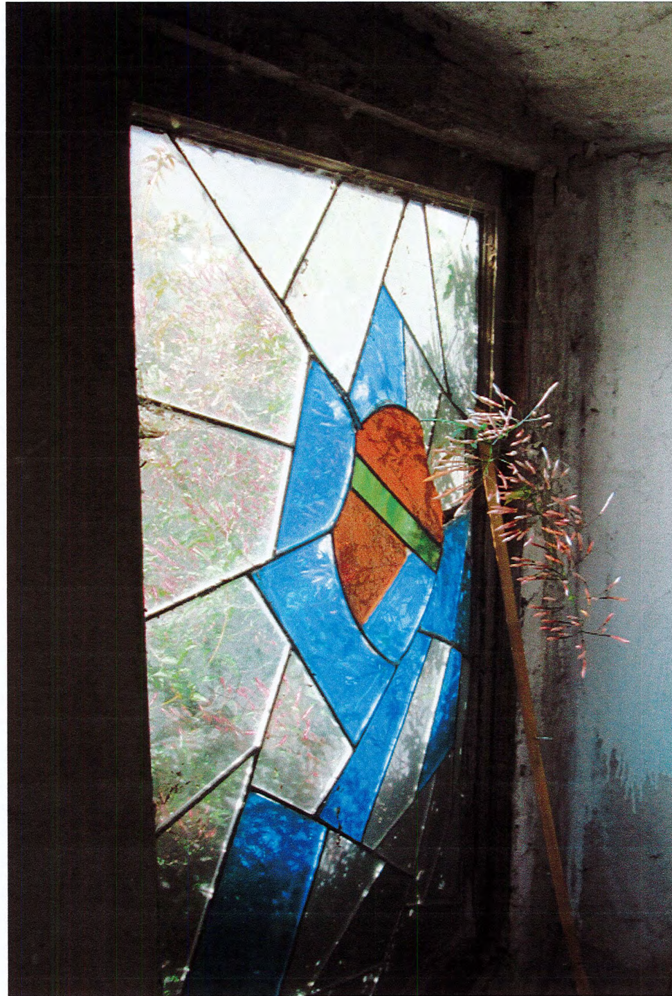
Stained glass front (west side - needs restoration)
