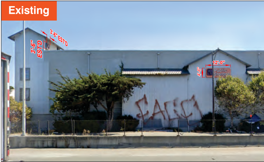
WEST ELEVATION BLDG C - STORAGE REMOVE & DISCARD EXISTING OPEN FACE CL SIGN
