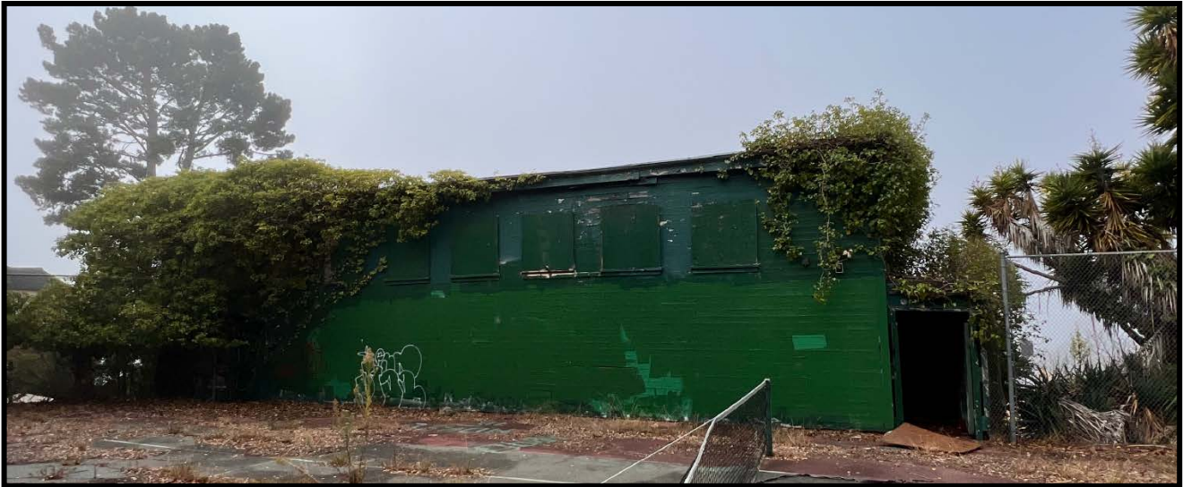
Figure 7: Subject property, gymnasium, east elevation, rehabilitation needed (2022).
