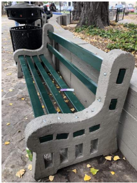
Benches - Repair concrete, replace wood
