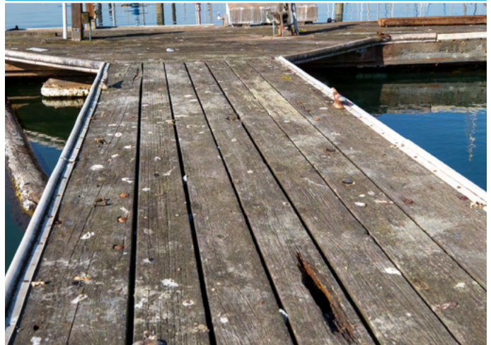
Deteriorated Marina Dock
