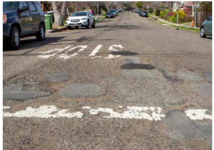
Street Pavement Damage
