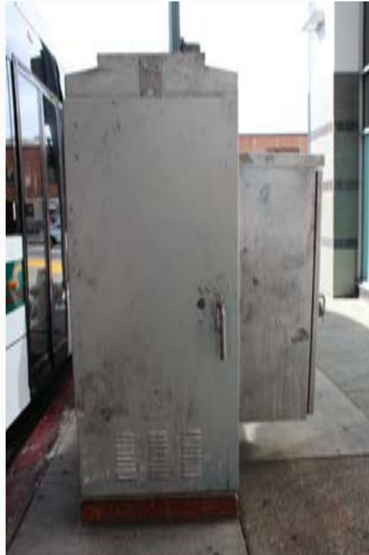
Location: Allston Way/Shattuck Ave.
