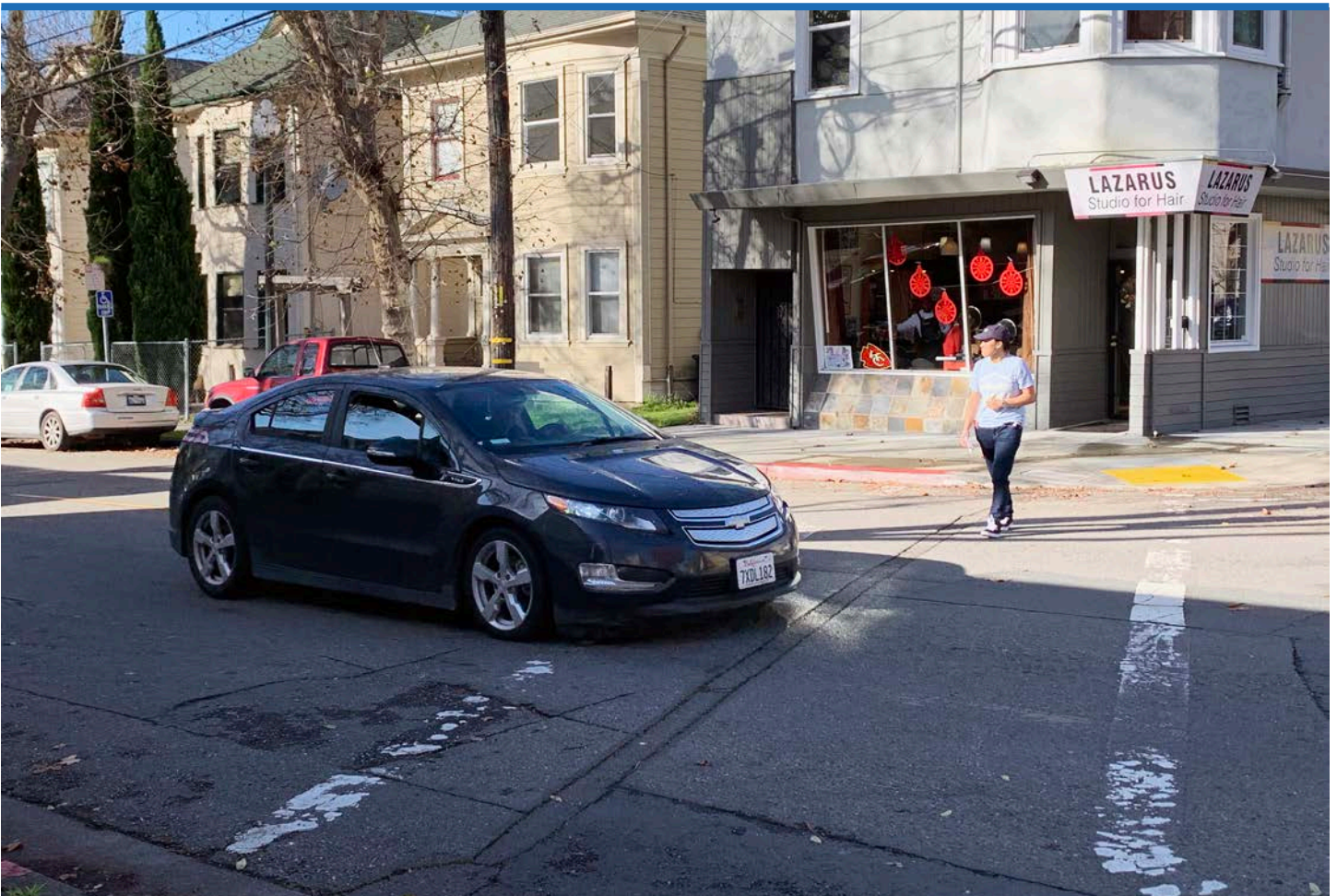
This pedestrian crossing at Alcatraz Avenue and King Street has faded crosswalk markings and worn pavement, which may make crossing the street more challenging.
