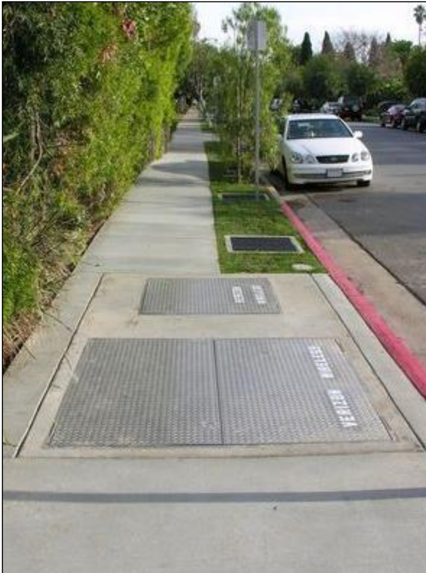
Figure 3: Flush-to-grade underground equipment vault.
