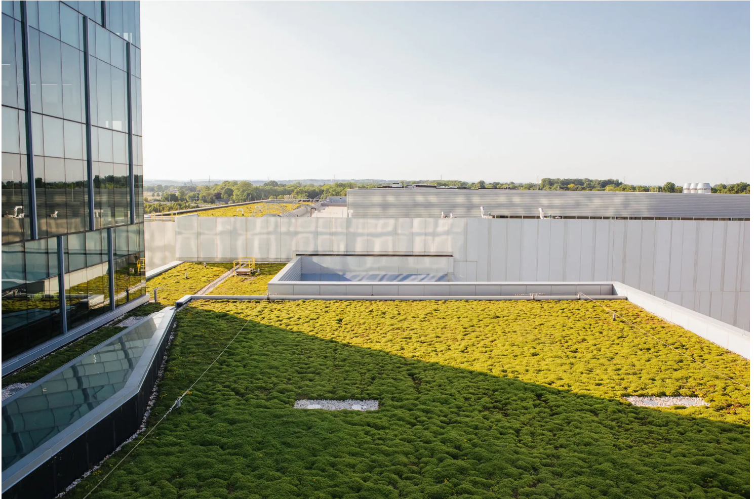
A green roof at the Air Products headquarters. Michelle Gustafson for The New York Times
