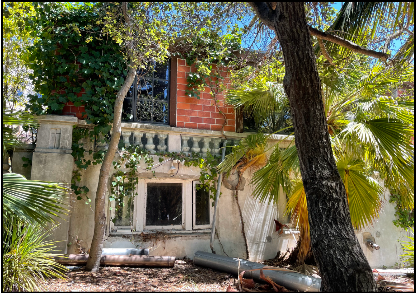
Figure 5: Subject property, west elevation of addition off west terrace. Upper level cafeteria/auditorium to be demolished to restore the southwest terrace. Game room below the terrace to be rehabilitated (2022).
