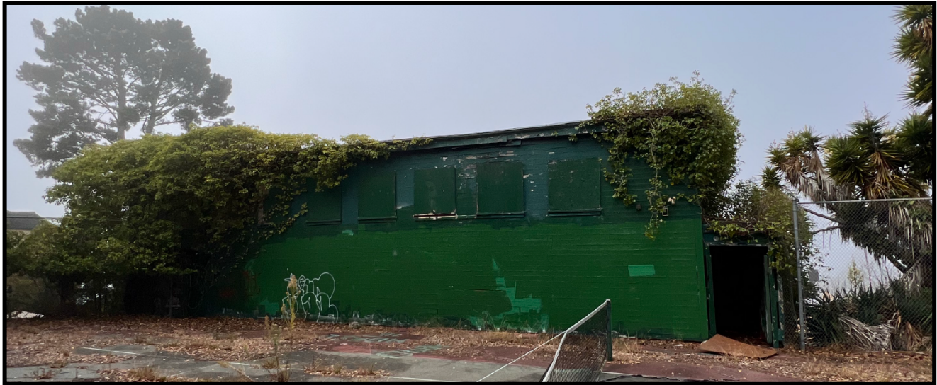
Figure 7: Subject property, gymnasium, east elevation, rehabilitation needed (2022).
