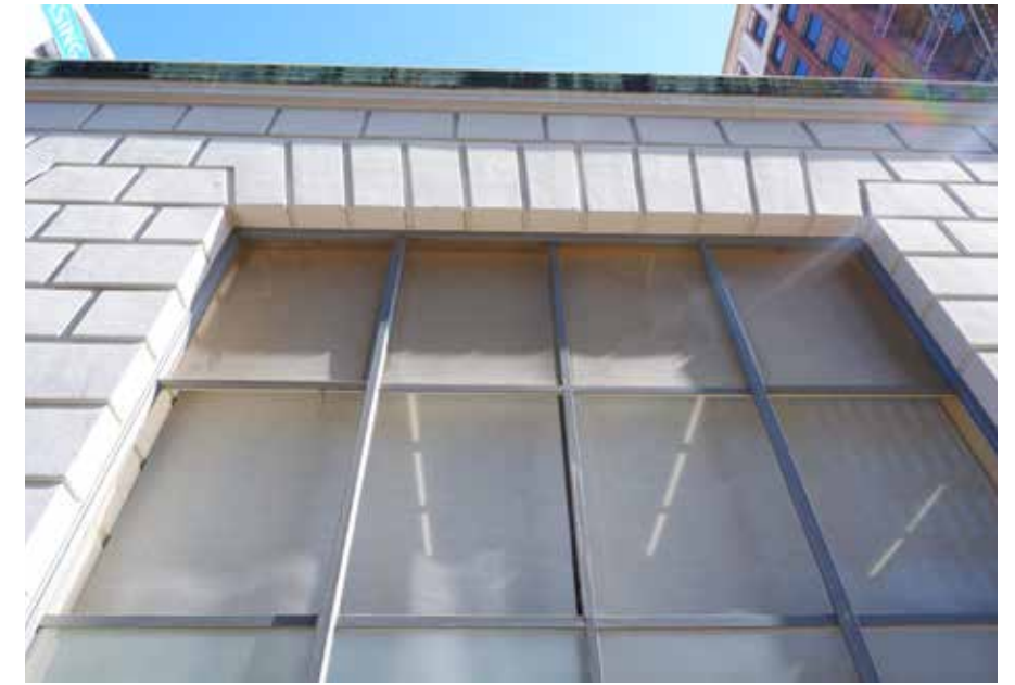
6. Closeup view of existing windows at area of work on Center Street.
