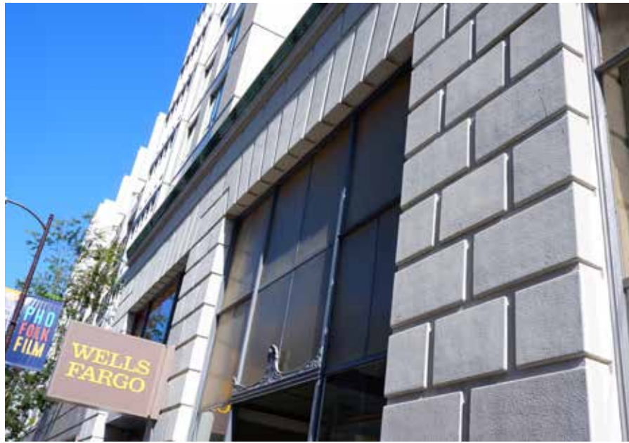
5A. Closeup view of transom window above existing pedestrian entrance on Center Street.
