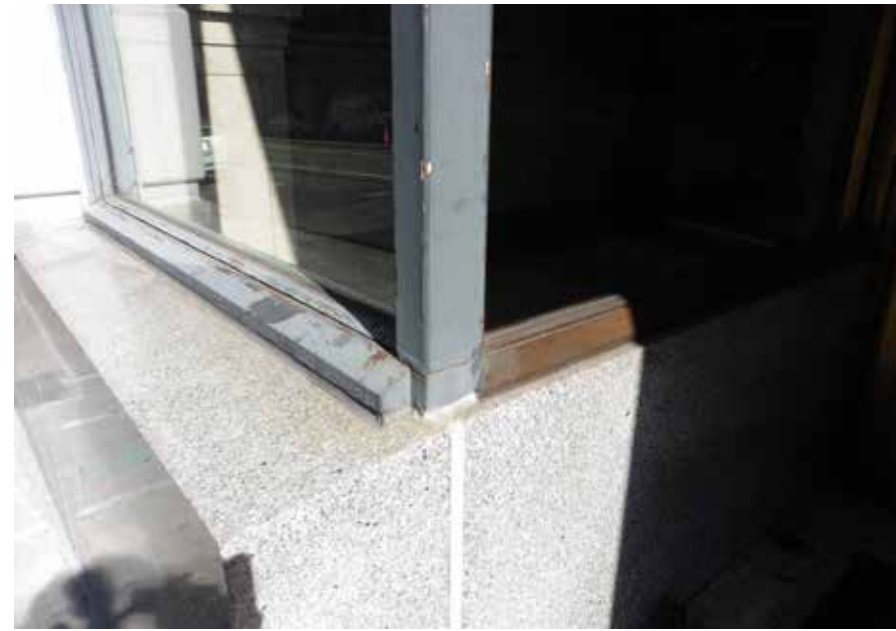
5B. Closeup view of storefront glazing system sill at existing entrance on Center Street.
