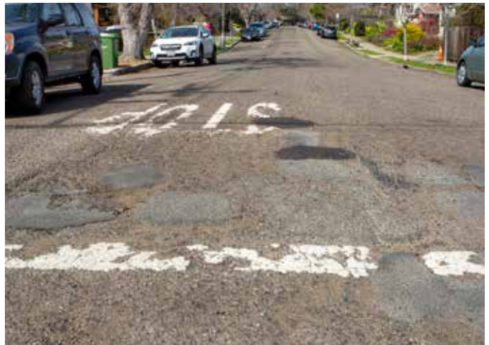
Street Pavement Damage
