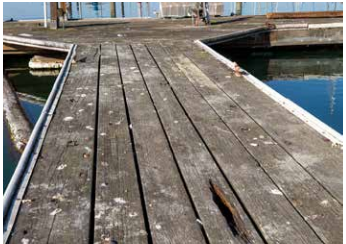
Deteriorated Marina Dock
