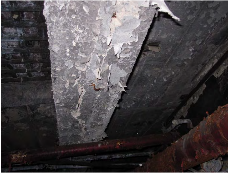
Figure 16. Serious crack in major beam in First Floor at Basement
