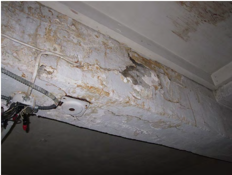
Figure 17. Crack in major beam in First Floor at Basement
