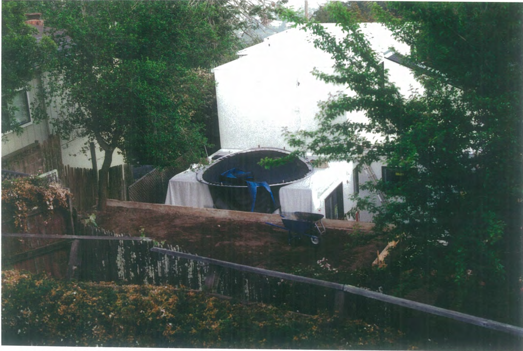
— PHOTO OF 1449 GUILLY PERLE BLVD. REAR YARD BEFORE FINAL CONCRETE POUR AND BEFORE THE PROTECTED LIVE OAK ( ON THE LEFT) WAS CUT DOWN.
