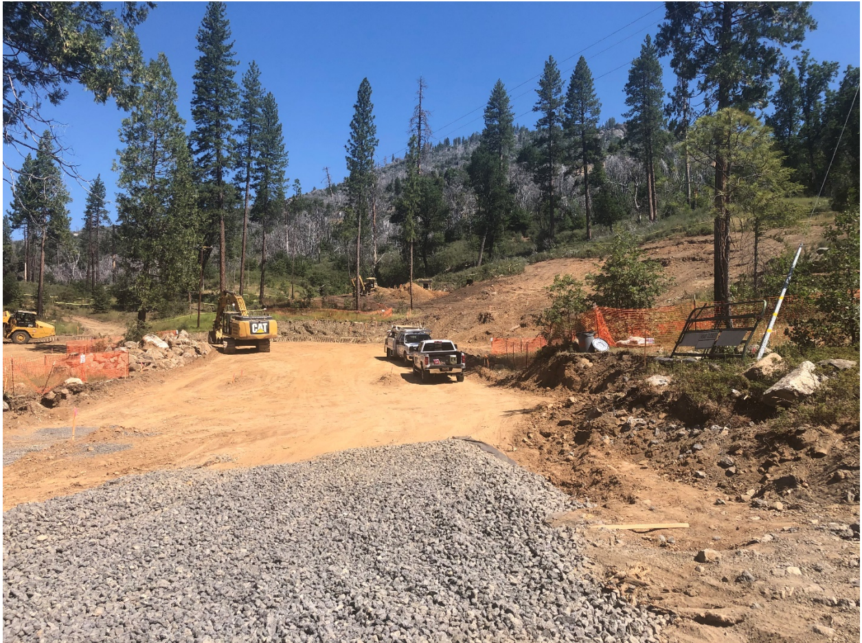
Staff Camp from Hardin Flat Road at entrance to new Parking Lot
