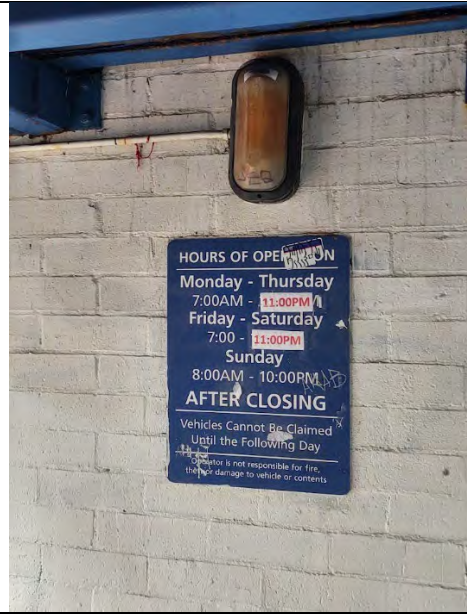
Broken light in stairwell above sign
