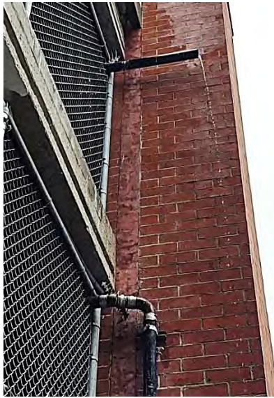
Missing drainage downspout
