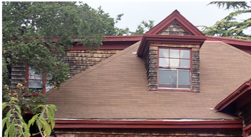
Figure 8. Front dormer in the original hip roof. Behind is the second story created in 1925.
