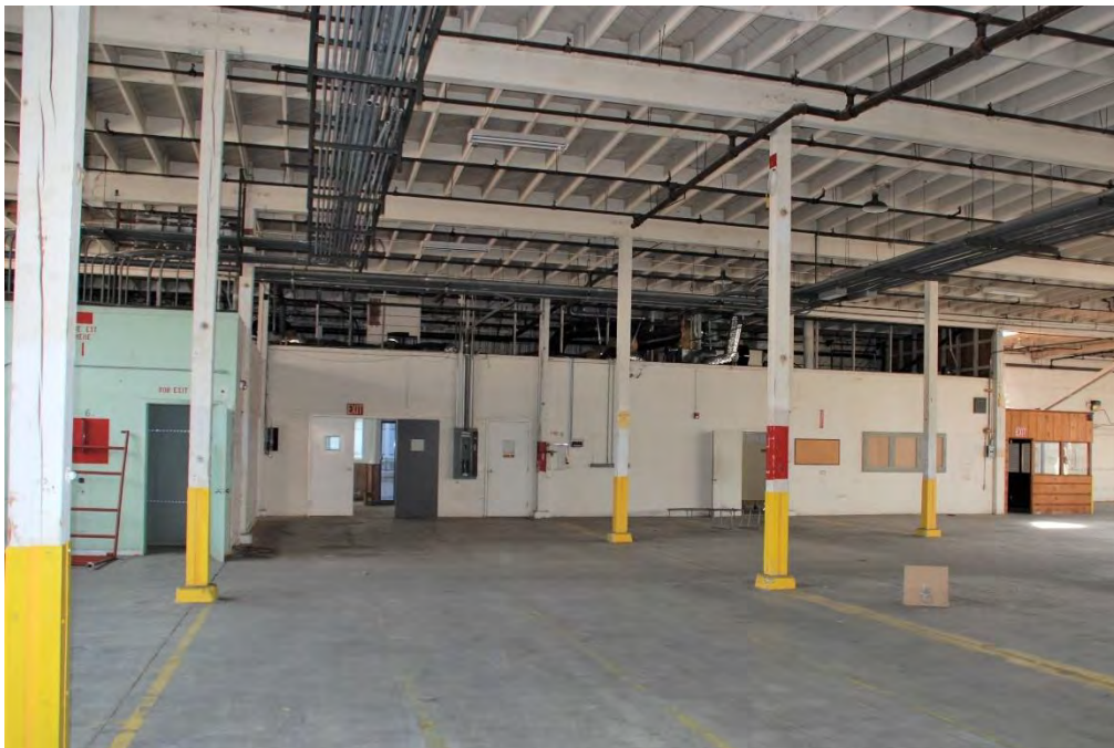
Figure 27. East warehouse building, interior of main space, view east toward enclosures: utility room, foyer, restroom, and office.
