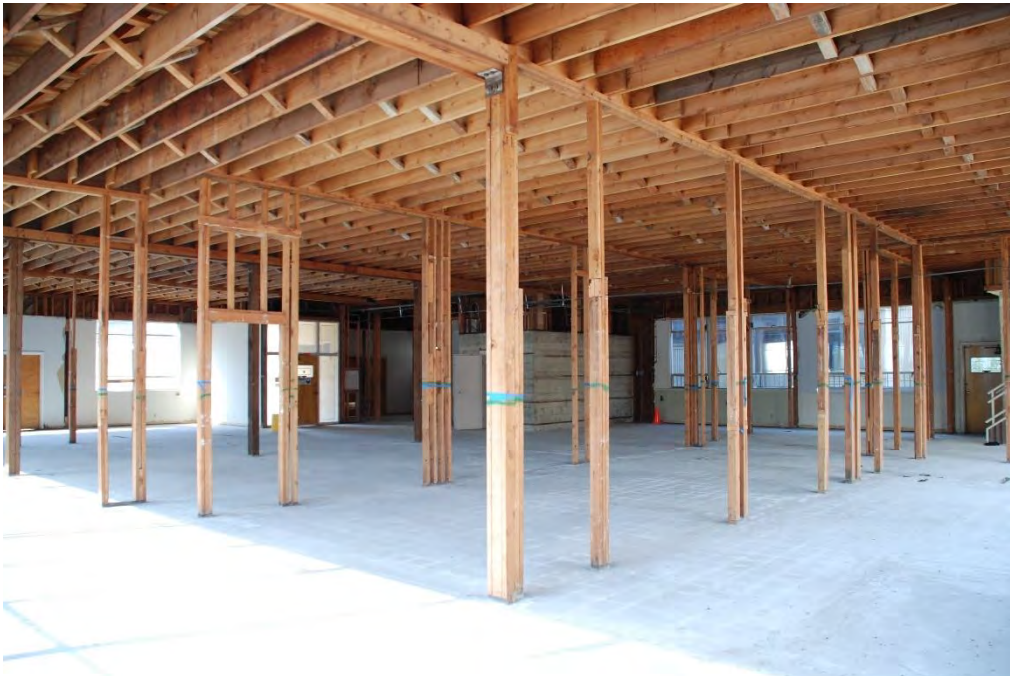
Figure 9. Office building, first floor interior, view southwest. Concrete safe in center background.
