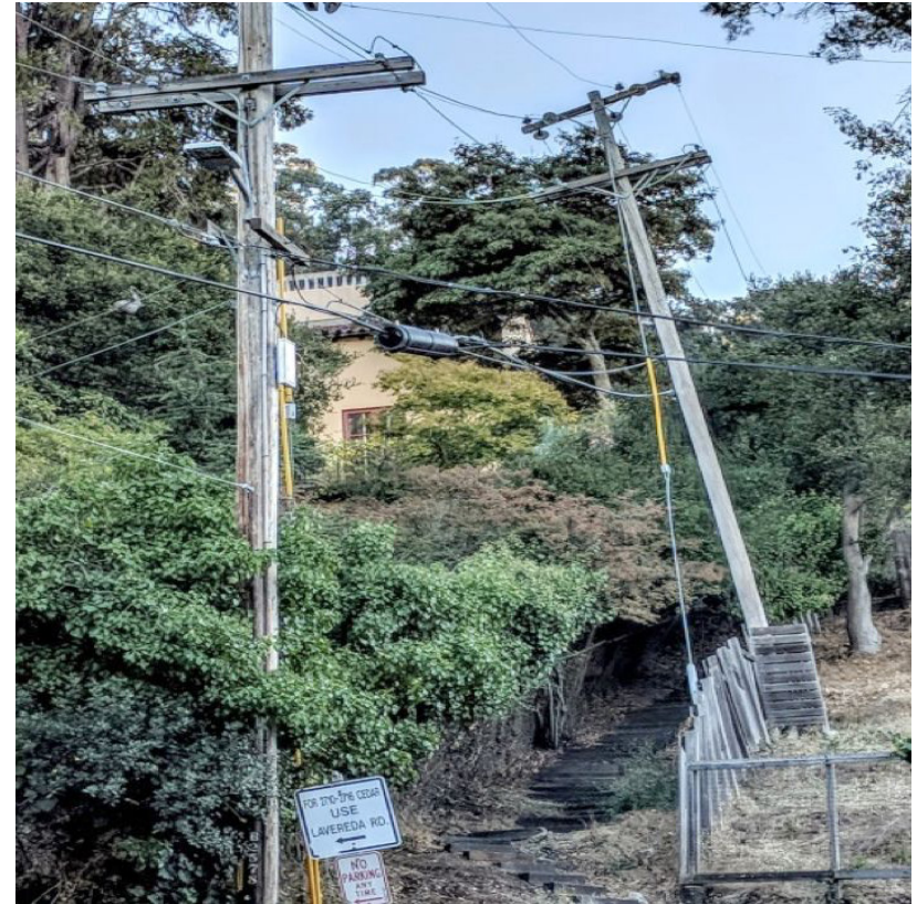
Overhead wires are a safety concern in Berkeley. Photo: Berkeley City Council Report
