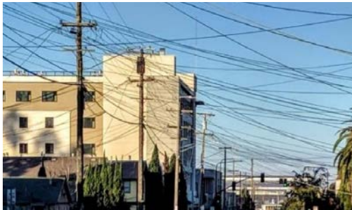
Dangerous overhead wires
