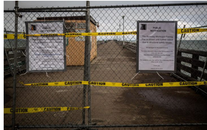
The pier is an example of deteriorated and unsafe infrastructure.
