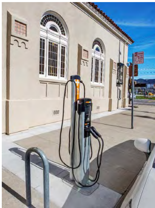
EV Charging Stations at the Mental Health Services Building
