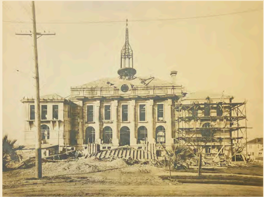
Figure 4.28 Berkeley City Hall under construction. Source: Bancroft Library, University of California, Berkeley.
