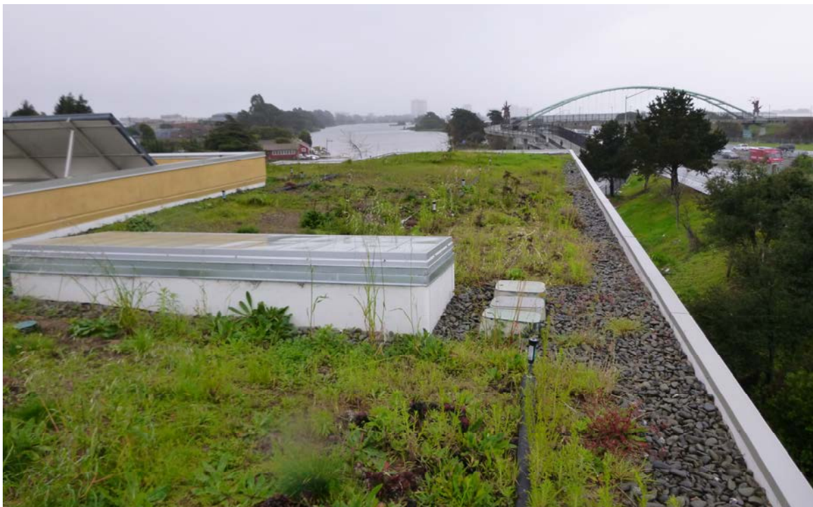
Figure 8 – The green roof at the City of Berkeley's Dona Spring Animal Shelter.
